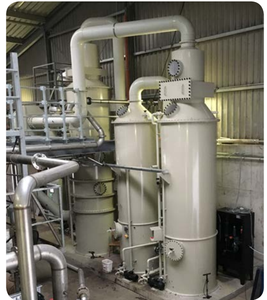
Ammonium-Strippungsanlage (Fa. BYOSIS)
