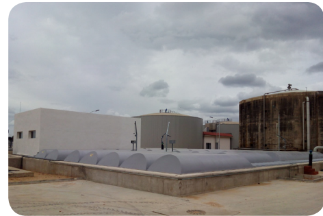
Example: Sewage treatment plant Badajoz / ES with BIOMOX® CFR
