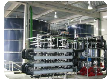
*) Mechanical-biological waste treatment
