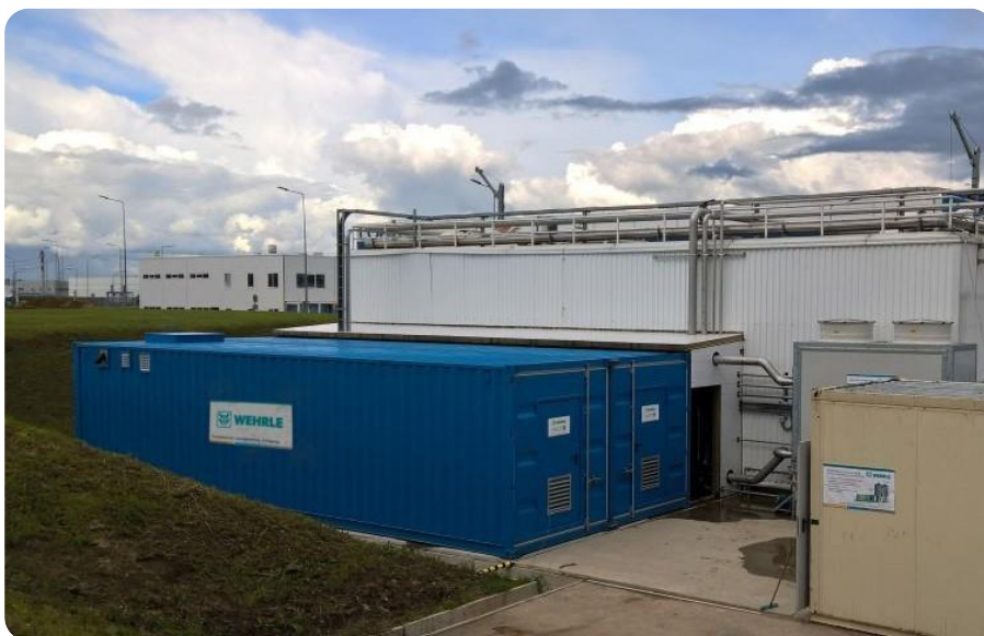
1) Finished Zero Liquid Discharge (ZLD) plant with bioreactor in the background and ultrafiltration and reverse osmosis containers in the foreground.
